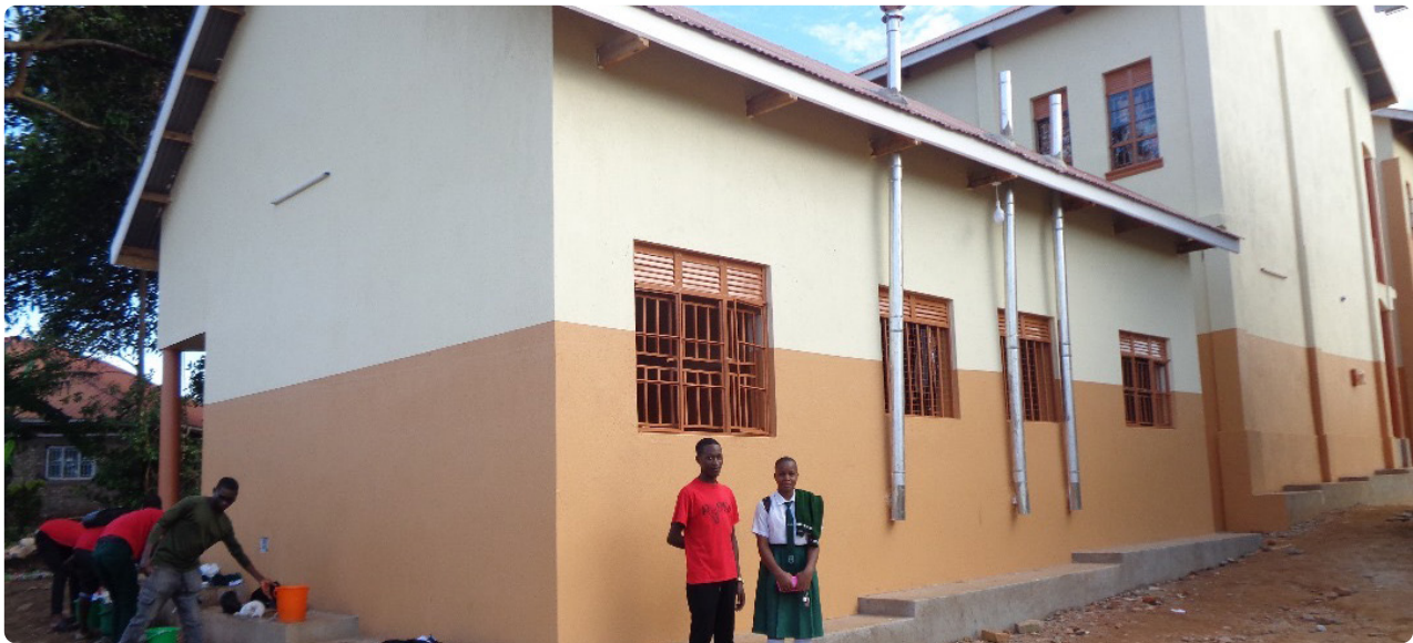
Ventilation and exhaust system of the new kitchen building
